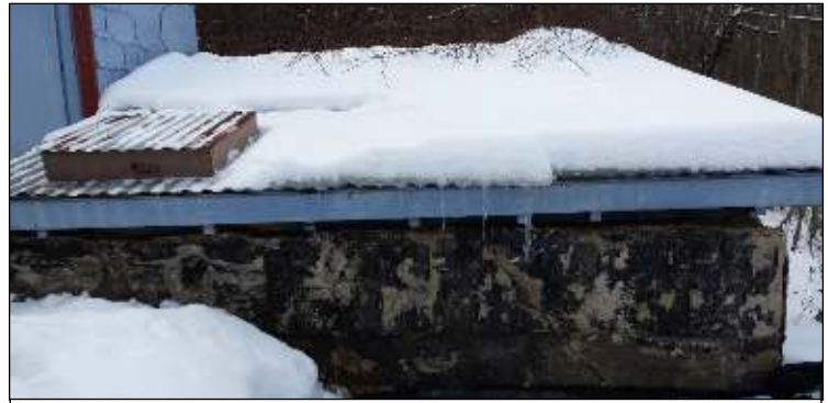
Photo showing the poor condition of the Watrous clearwell.
