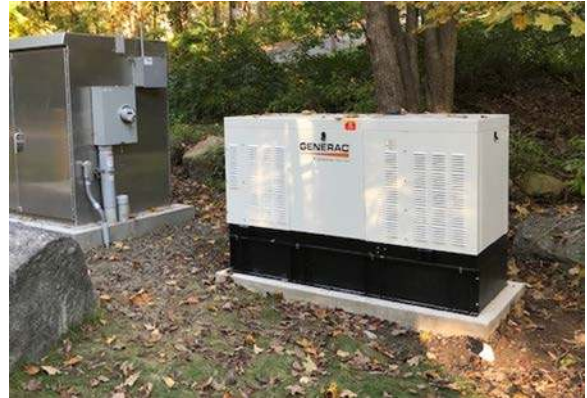
Briar Cliff Pump Station
